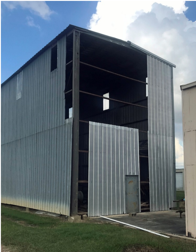
Figure 4. Damage to old foundation seed building used for storage.
