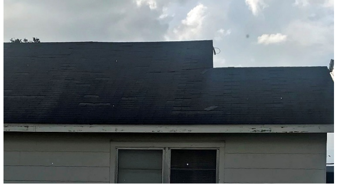
Figure 5. Roof damage on station building.
