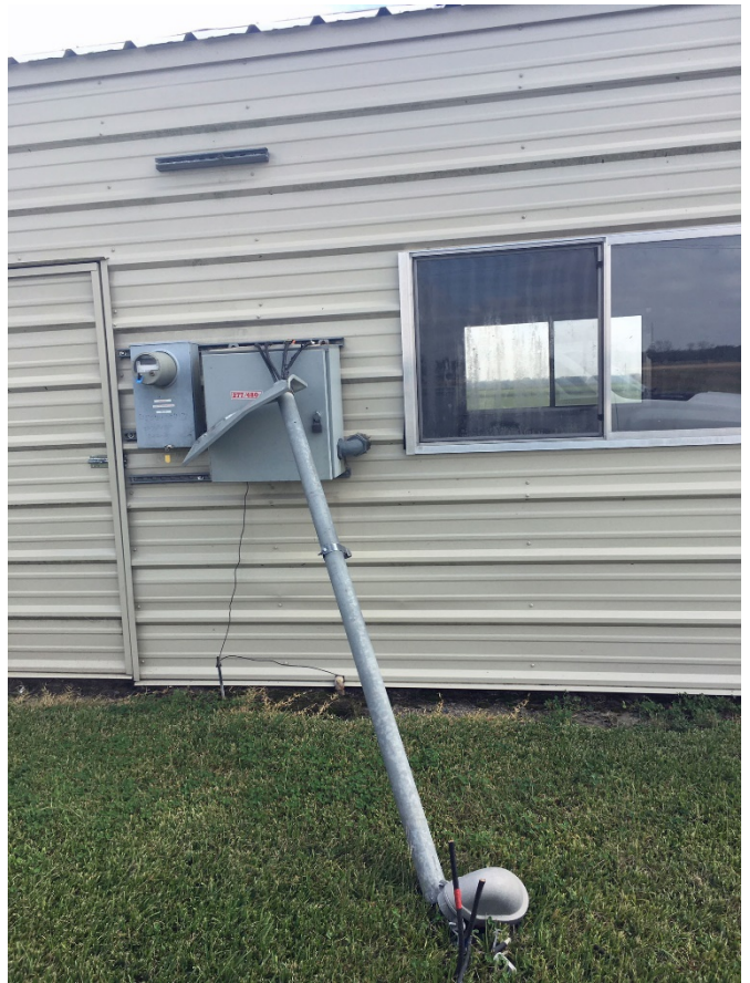
Figure 6. Downed power lines that feed station.
