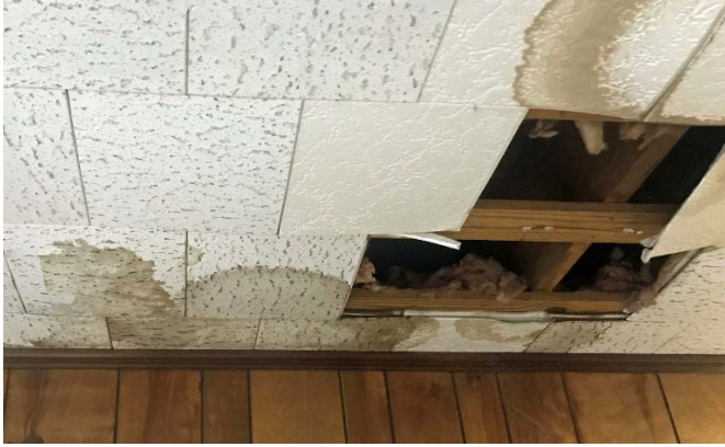
Figure 3. Water damage to Agronomy lab.
